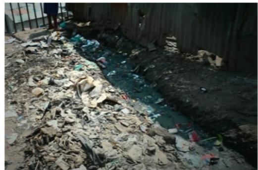
Poor sewerage and water drainage
